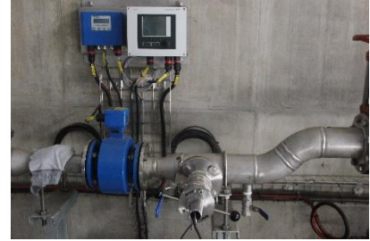
Darling WWTW: Sludge Flow Meter & inline Turbidity Meter
