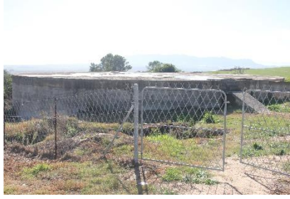
2.810 MI Klipkop Reservoir
