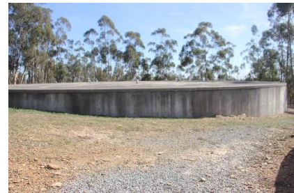
4.582 MI Moorreesburg Reservoir No. 2
