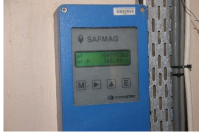
Rustfontein Booster PS Flow meter
