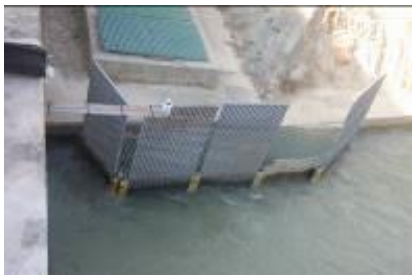
Inlet to raw water PS from Voëlvlei Canal
