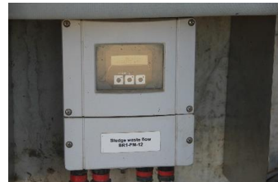
Malmesbury WWTW: Sludge take-off Flow Meter
