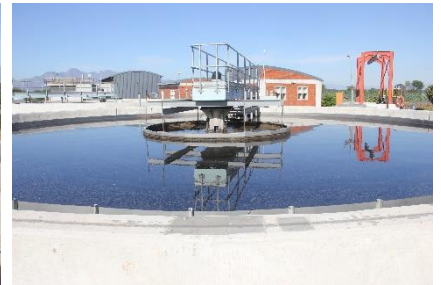
Secondary Settling Tanks
