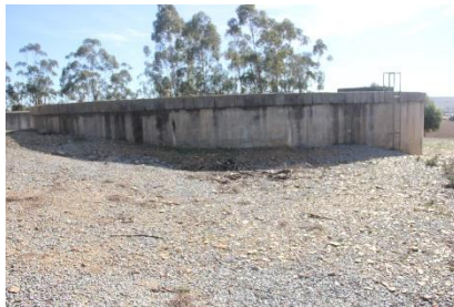
1.036 MI Moorreesburg Reservoir No. 1
