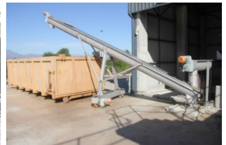
Conveyor and Skip for Belt Press
