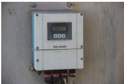
Malmesbury WWTW: Incoming Flow Meter
