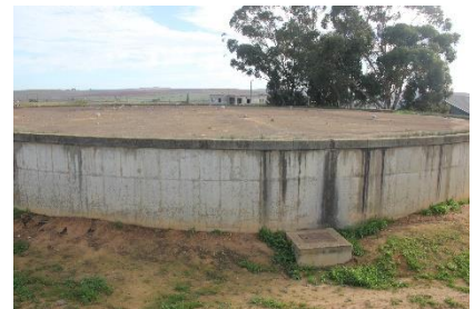
5.138 MI Wesbank Reservoir No. 3
