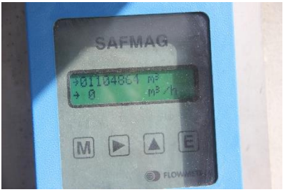
Riebeek Valley WWTW: Inflow Meter
