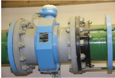
Darling PS Flow meter
