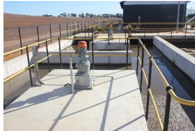
Bio Reactor: Two anaerobic zones with mixers
