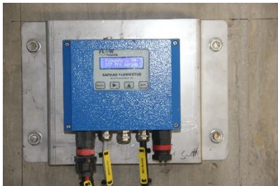
Darling WWTW: Service Water Flow Meter
