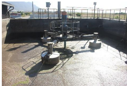
Aerobic Digester with floating aerator
