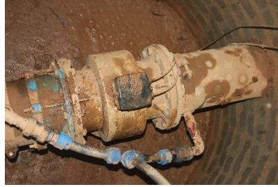
Chatsworth Reservoir outlet (Dia 350)
