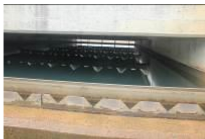
Horizontal flow sedimentation tanks
