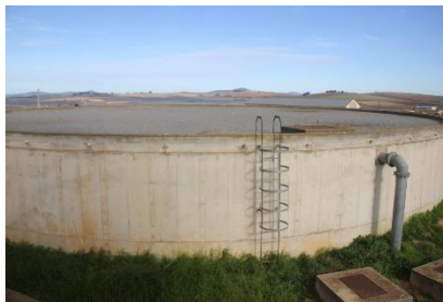
3.322 MI Wesbank Reservoir No. 2
