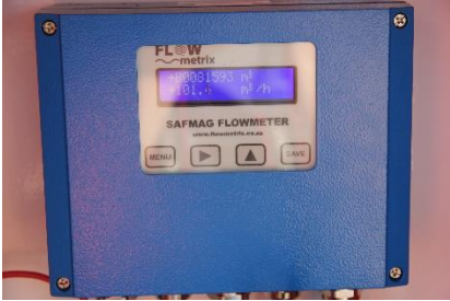
Moorreesburg WWTW: Incoming Flow Meter
