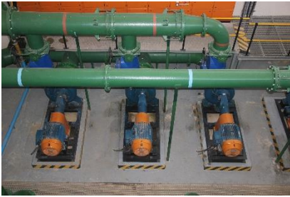
Raw Water PS at Swartland WTW
