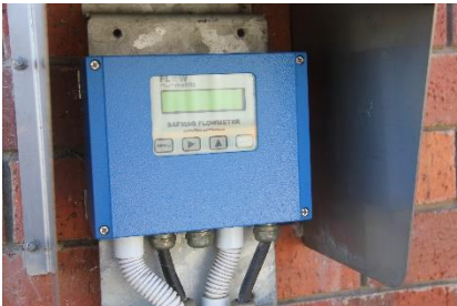
Riebeek Valley WWTW: Final Flow Meter
