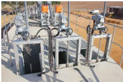
Inlet Works (Hand-rake bypass screen and two rotary mechanical drum screens)
