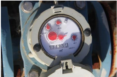
Moorreesburg WWTW: Re-use (irrigation) Bulk Water Meter
