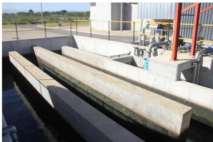
Chlorine contact channel
