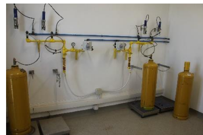
Disinfection with chlorine gas.
