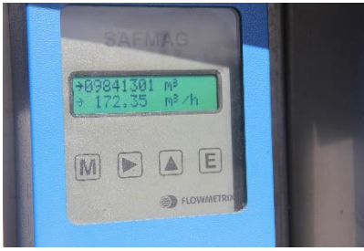
Riebeek Valley WWTW: Flow meter for RAS PS
