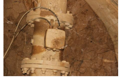
Chatsworth Reservoir outlet (Dia 200)
