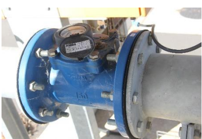
Riebeek Valley WWTW: Irrigation Meter
