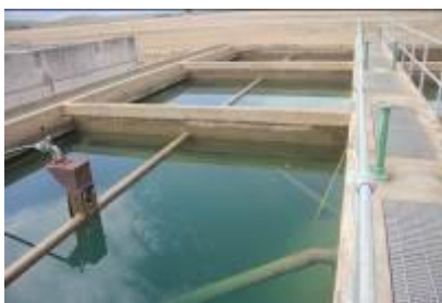
Vertical flow sedimentation tanks
