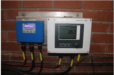
Moorreesburg WWTW: Flow meter & Turbidity Meter
