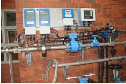
Riebeek Valley WWTW: Poly and sludge Flow meters
