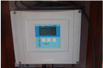
Moorreesburg WWTW: Final Effluent Flow Meter
