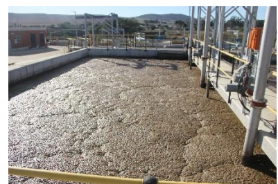
Bio Reactor: Aerobic zone (Bubble Aeration)
