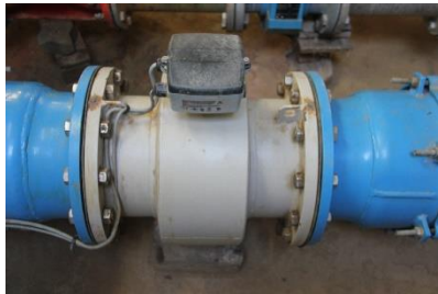
Riebeek Kasteel Reservoirs Outflow (Dia. 250)
