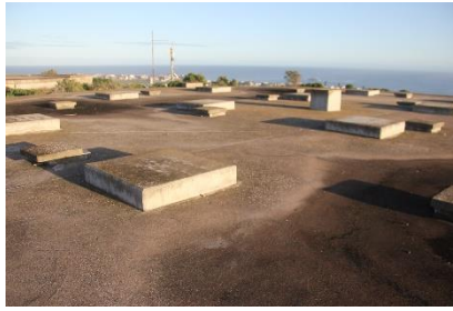
1.822 MI Yzerfontein Old Reservoir
