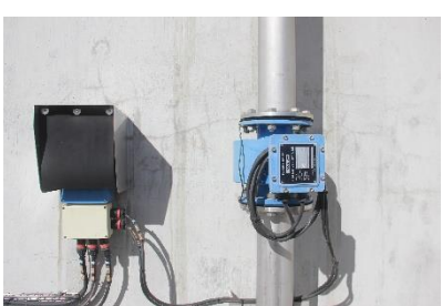
Riebeek Valley WWTW: Flow meter for Aerobic Digester
