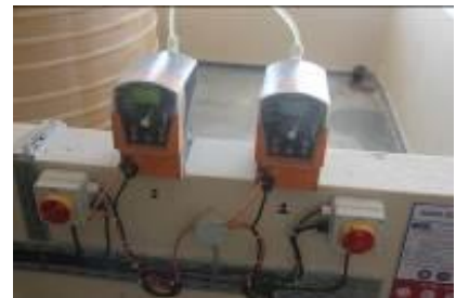
Sudfloc 3870 dosing pumps (Duty/Standby)
