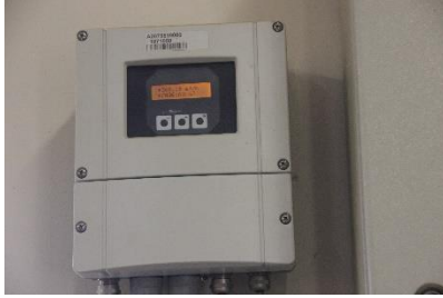
Swavelberg Booster PS Flow meter
