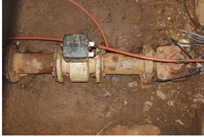
Koringberg Reservoir inlet (Dia. 100)
