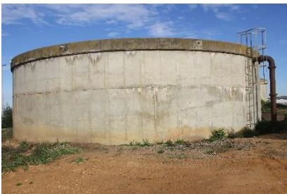
0.988 MI Wesbank Reservoir No. 1
