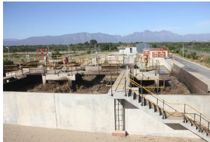
Activated sludge bioreactor
