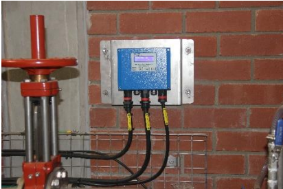
Moorreesburg WWTW: Poly Flow Meter
