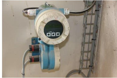
Yzerfontein PS Flow meter
