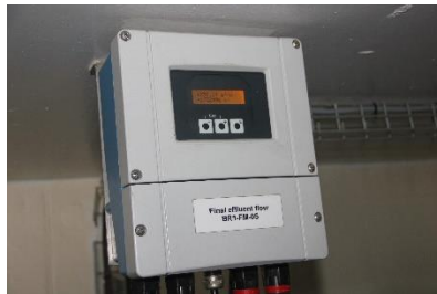
Malmesbury WWTW: Final Effluent Flow Meter
