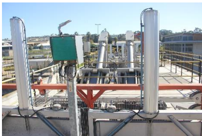
Inlet works with hand raked screens
