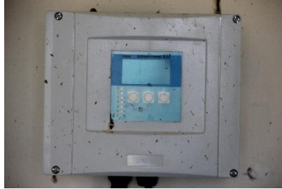
Darling WWTW: Final Effluent Flow Meter
