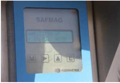
Riebeek Valley WWTW: Flow meter for WAS PS
