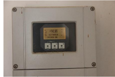
Moorreesburg PS Flow meter
